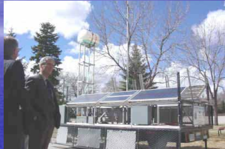
Solar powered pumps
