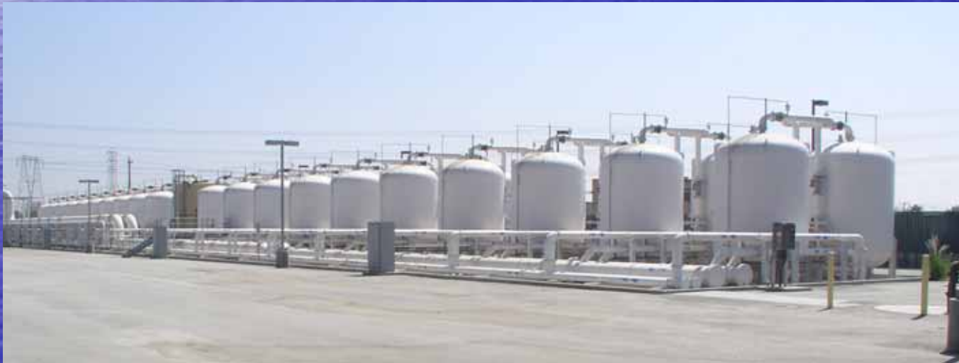
Whittier Treatment Plant Bowlin
